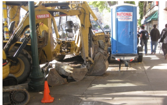
(Construction on Shattuck temporarily narrows the sidewalk width, making it harder and more dangerous for pedestrians to travel through the street)
